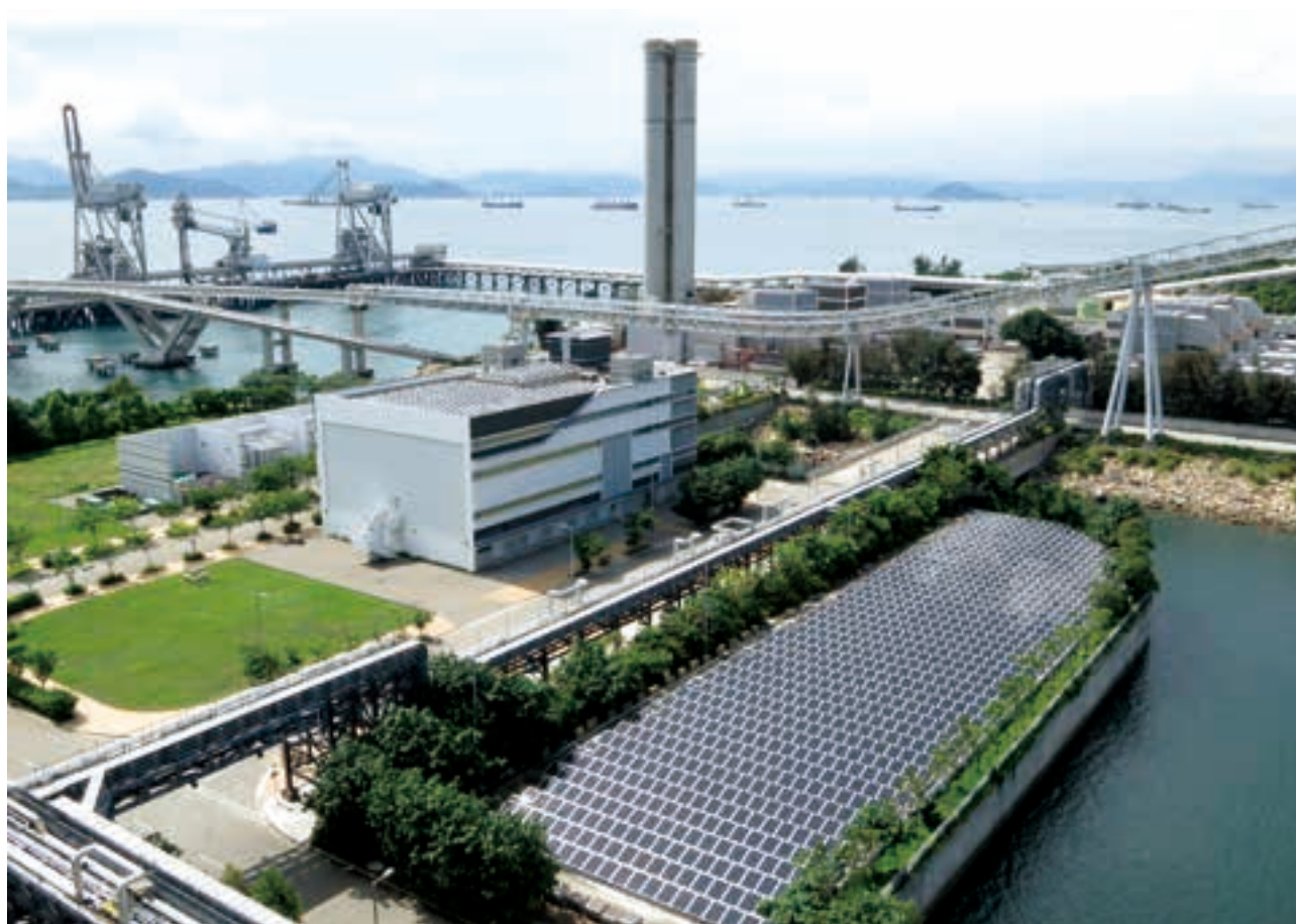
HK Electric's solar power system at Lamma Power Station, the largest of its kind in Hong Kong, further expands its installed capacity to 1MW.
